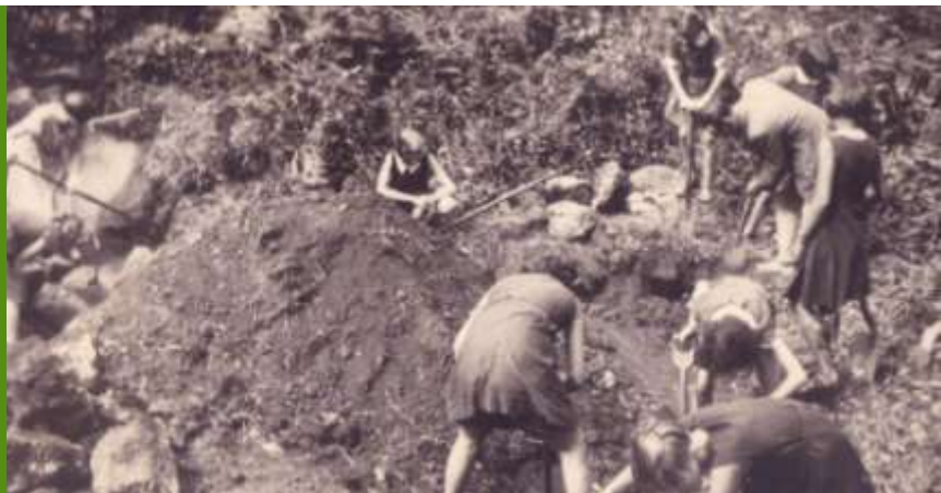
Pupils at the Garden School helping to dig the foundations for the new swimming pool, c1932. From The White Family Collection (Ref: DC/WF/4/251).
